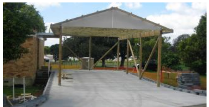
The new Ambulance Bay will be complete in the next couple of weeks
